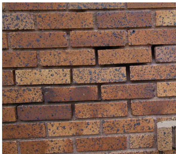
Eroded mortar joints should be repointed with matching mortar and joint tooling
