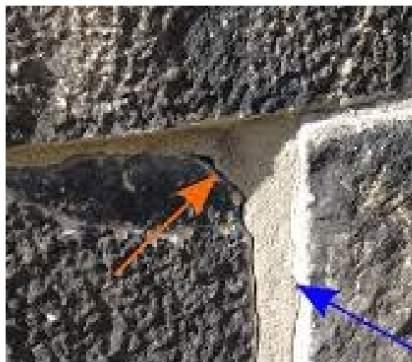
Mortar separating from brick or stone should be repointed.
