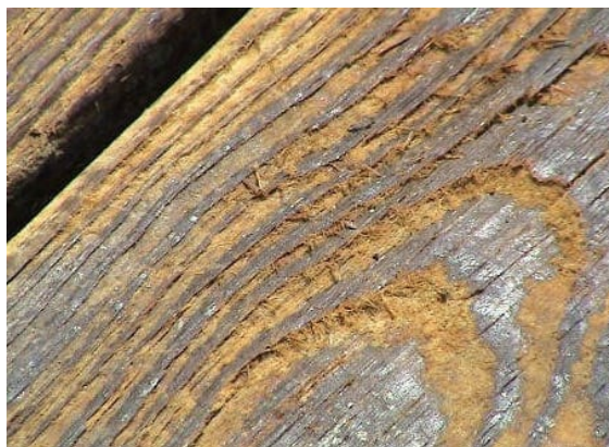
Wood deck damaged by pressure washing
