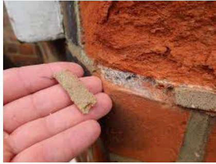
Cracking from overfilled mortar
