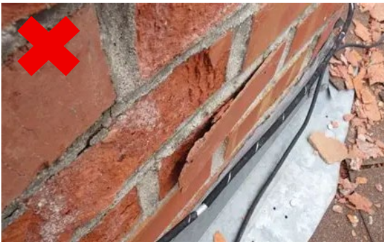
Spalling occurs when water penetrates the surface of the brick and then freezes. Cement mortars trap moisture and make it difficult for the brick to dry out.
