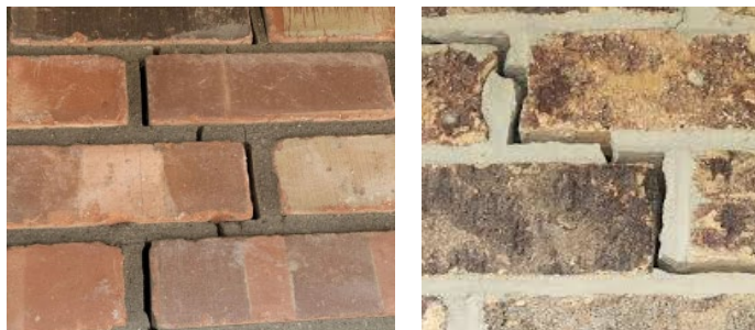
Examples of mortar joint failure
