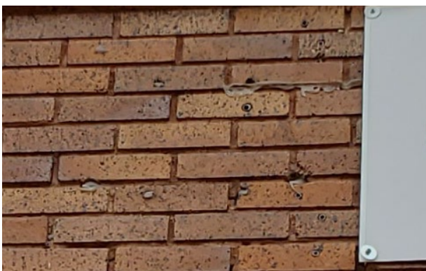
Holes in brick or stone are very difficult to patch. Holes drilled for the signs of new occupants add up over the lifetime of a historic building.
