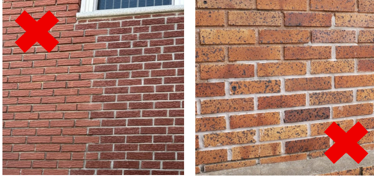
Poor matches for mortar color and tooling
