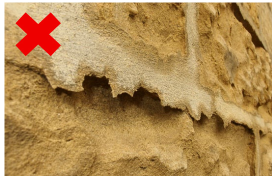
Sandstone damaged by cement mortar that is harder than the stone. As the building settles, tiny cracks form in the stone rather than in the mortar. Water penetrates the cracks and then expands when it freezes, cracking the stone.
