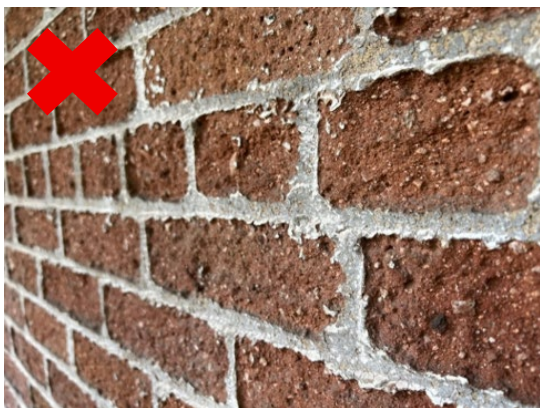
Brick damaged by aggressive pressure washing
