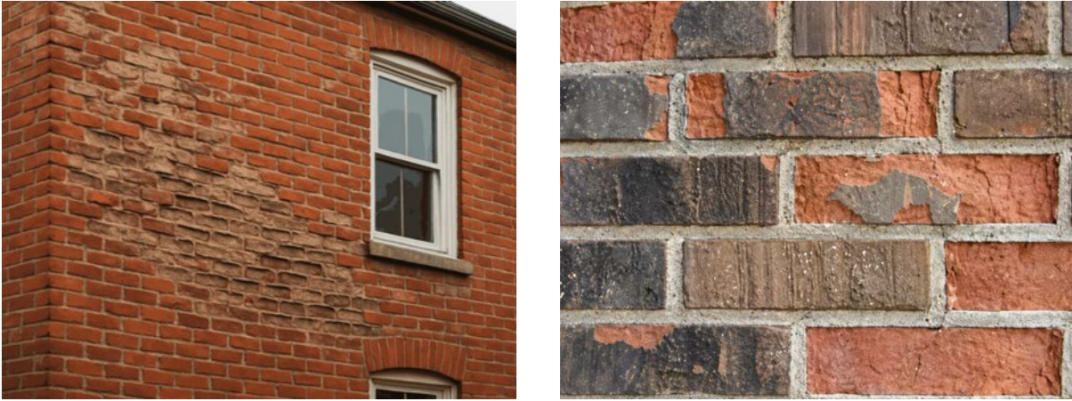
Spalling occurs when water penetrates the surface of brick or stone and then freezes. Cement mortars accelerate this process because it keeps the brick from drying out.
