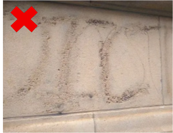
Limestone wall damaged when graffiti was removed with a pressure washer, etching the letters permanently onto the building
