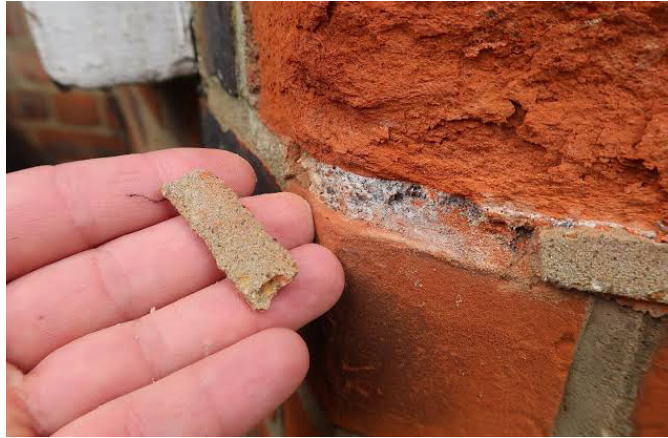
Cracking from overfilled mortar
