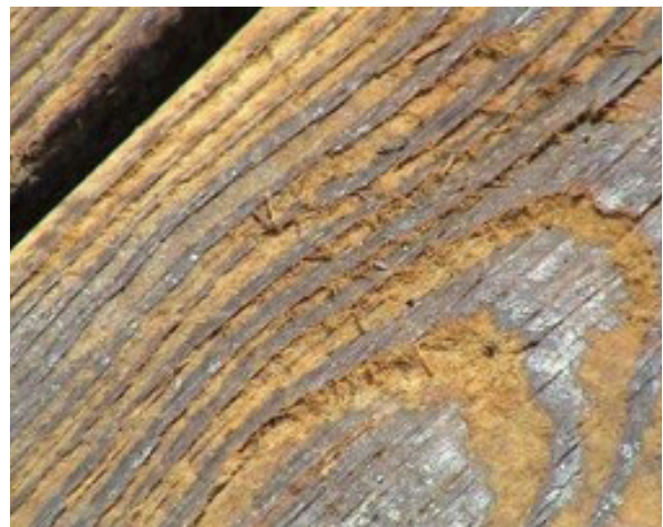
Wood deck damaged by pressure washing
