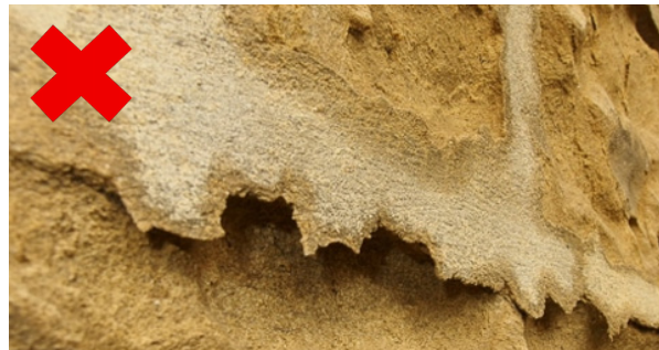
Sandstone damaged by cement mortar that is harder than the stone. As the building settles, tiny cracks form in the stone rather than in the mortar. Water penetrates the cracks and then expands when it freezes, cracking the stone.
