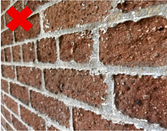
Brick damaged by aggressive pressure washing
