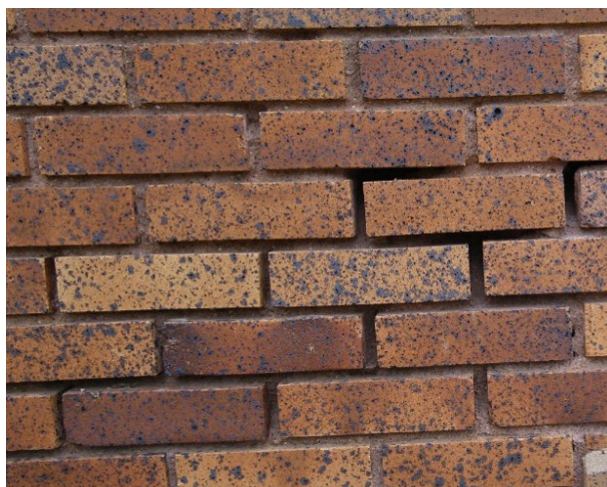
Eroded mortar joints should be repointed with matching mortar and joint tooling.
