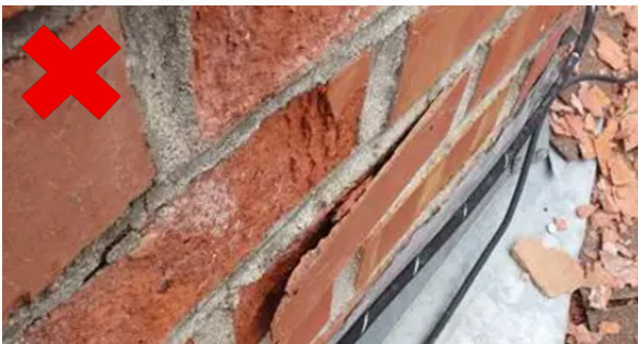
Spalling occurs when water penetrates the surface of the brick and then freezes. Cement mortars trap moisture and slow the brick's ability to dry out.
