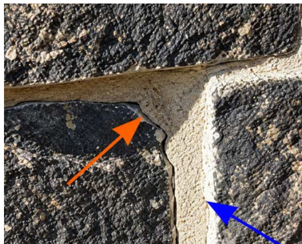
Mortar separating from brick or stone should be repointed.
