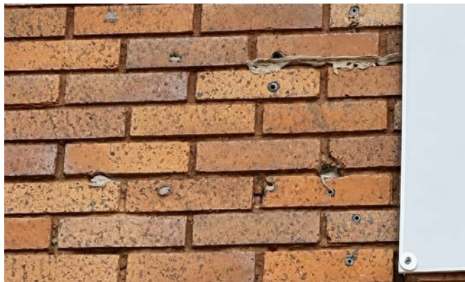
Holes in brick or stone are very difficult to patch. Holes drilled for the signs of new occupants add up over the lifetime of a historic building.
