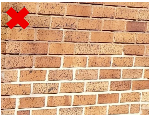
AVOID poorly matched mortar that has a different color and tooling pattern from the original mortar
